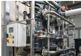
Water Filtration & RO Equipment
